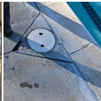
Cracked Skimmer To
