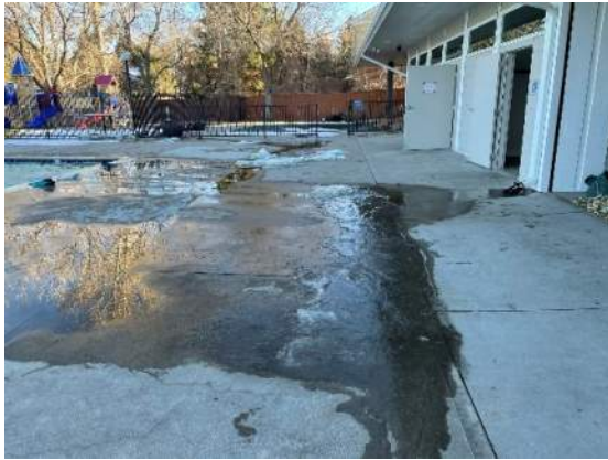
PONDING FROM DOWNSPOUTS
