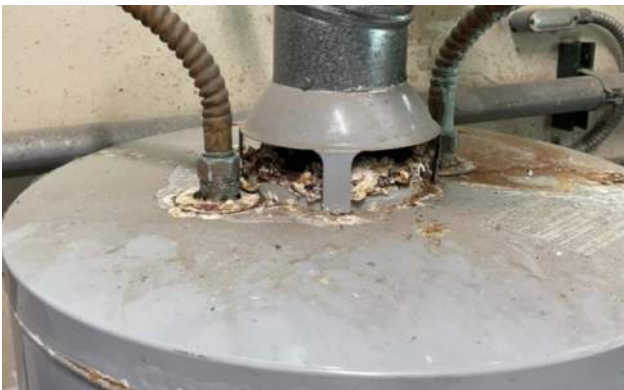
DOMESTIC WATER HEATER VENT CONNECTION
