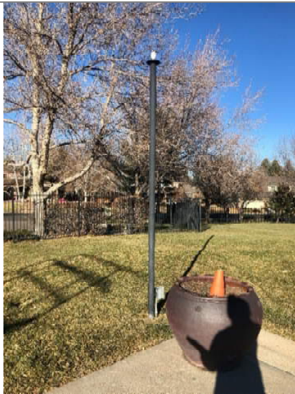
ROOM: Exterior - Pool Deck Existing Post-Top Area Light - Globe Missing
