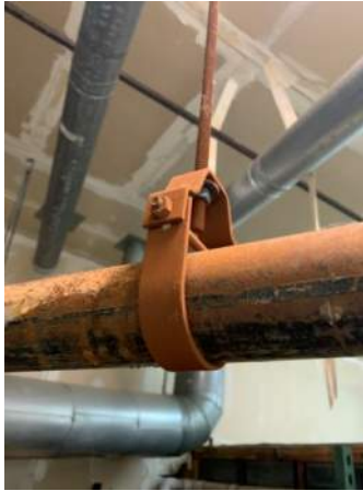
GAS PIPE AND HANGER CORROSION
