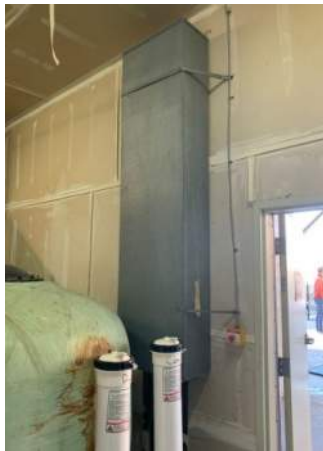
POOL EQUIPMENT ROOM CA OPENINGS AND EPO SWITCH
