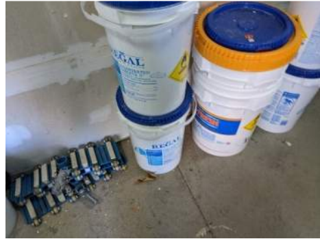
Chemicals in Pool Equip. Room
