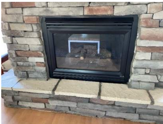
INOPERABLE FIRE PLACE
