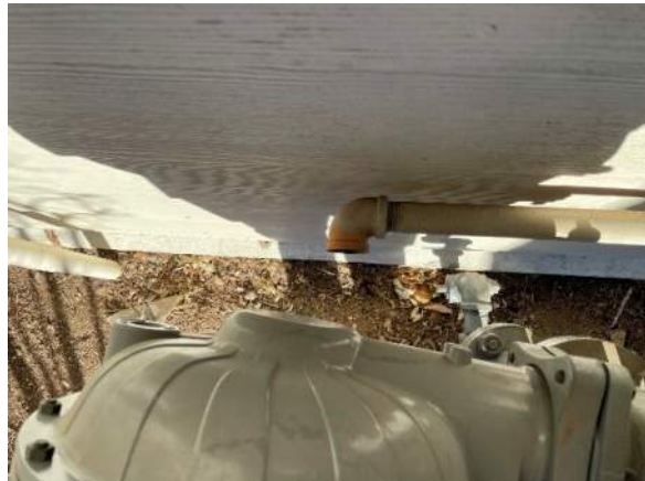
ABANDONED GAS VENT RELIEF PIPE
