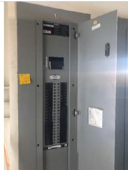
ROOM: Check-in Storage Existing Panel L2
