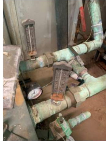
POOL BOILER PIPING CORROSION
