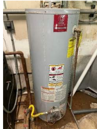
EXISTING WATER HEATER
