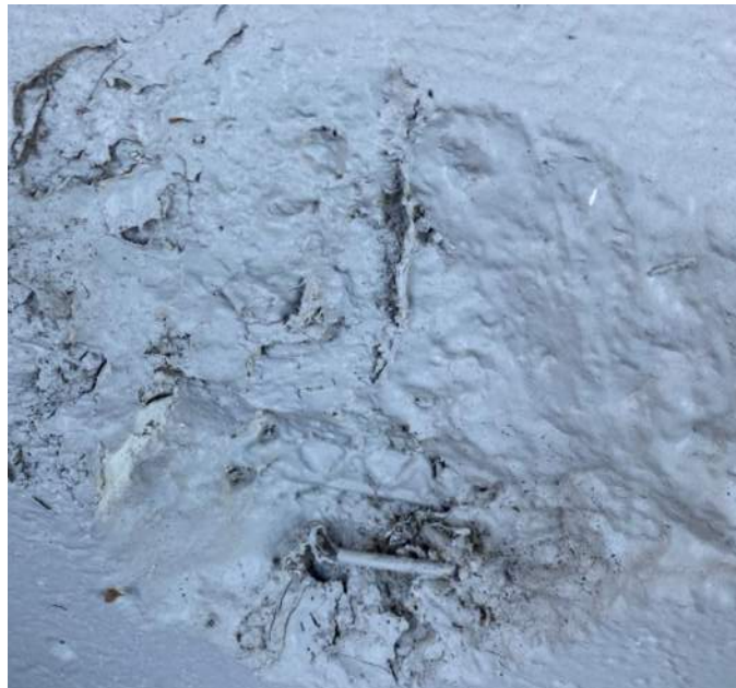
Photo 2: Exposed stem wall rebar
