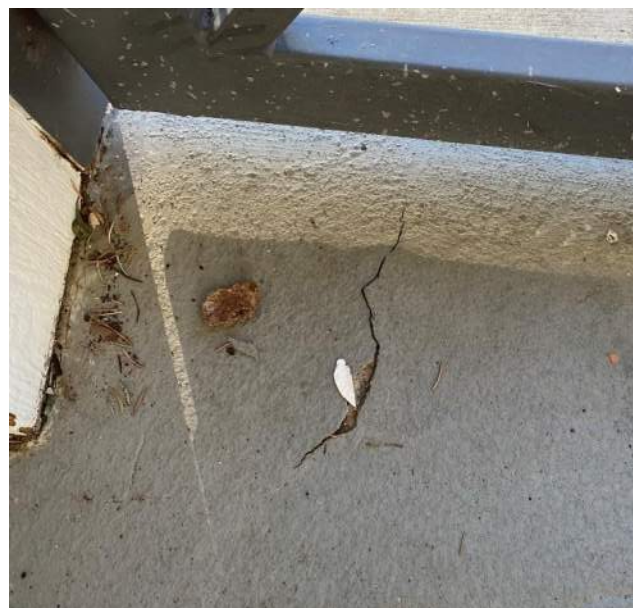
Photo 3: Cracking floor coating at central walkway
