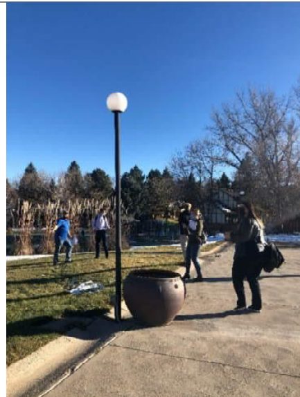
ROOM: Exterior - Pool Deck Existing Post-Top Area Light with Globe
