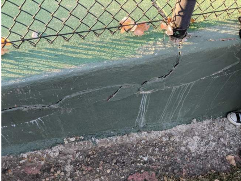
Photo 5: Spalling at east side of tennis courts
