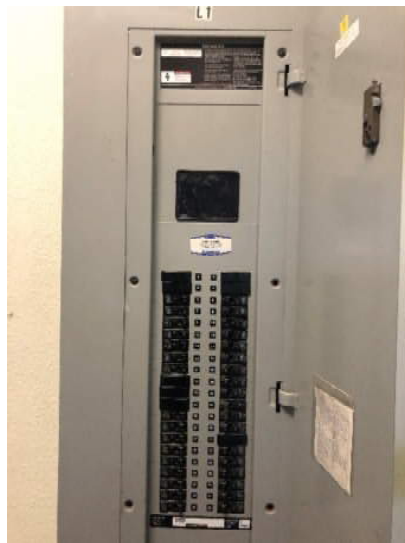
ROOM: Check-in Storage Existing Panel L1
