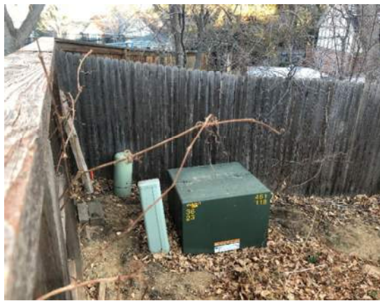
ROOM: Exterior Existing pad-mounted transformer service to pool building.
