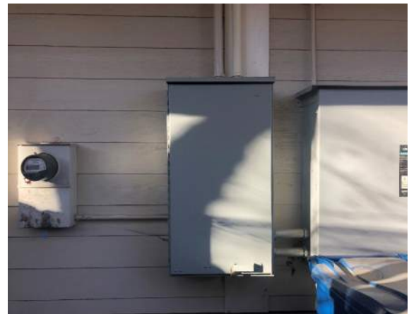
ROOM: Exterior (South side of Bathhouse) Existing Disconnect, CT, and Meter
