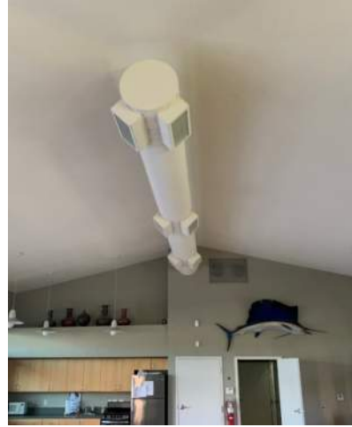
COMMUNITY ROOM SUPPLY DUCTWORK AND RETURN GRILLE
