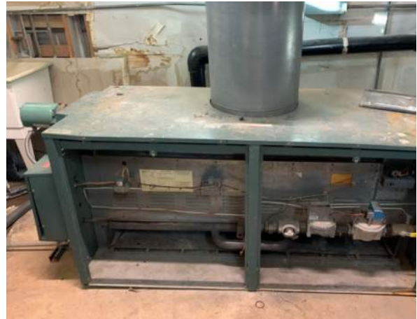
POOL HEATER AND ASSOCIATED FLUE
