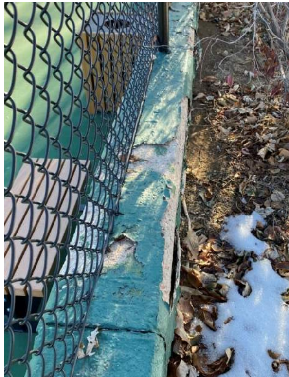
Photo 4: Coating failure at tennis court retaining walls
