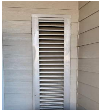
POOL EQUIPMENT ROOM COMBUSTION AIR LOUVER
