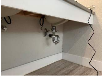
LAVATORIES NOT ADA
